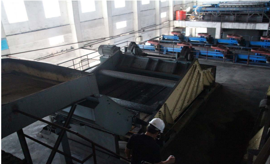
Figure 4 Jig (coarse coal separator) area with float cells in background
